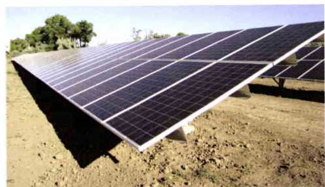
Aztec, NM Solar Field
